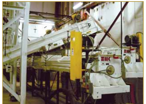
Installation of 3 - 16SWR-MS. The conveyors are moving pet food to the bagging operation.
