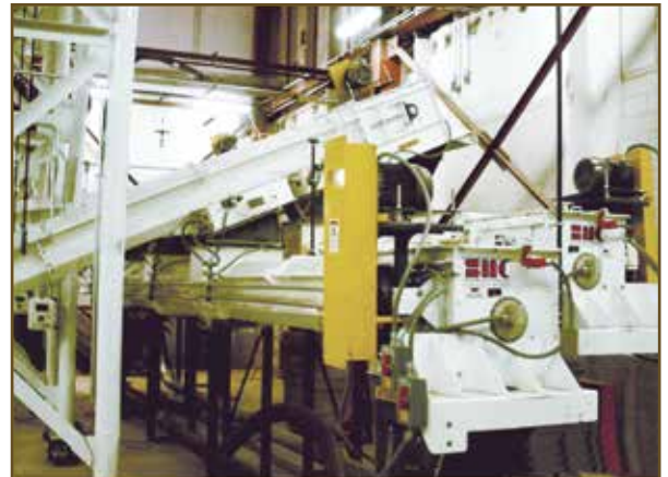
Installation of 3 -16SWR-PF. The conveyors are moving pet food to the bagging operation.
