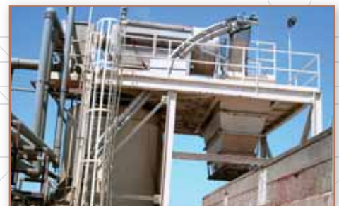
Double bend - tomato waste conveyor.
